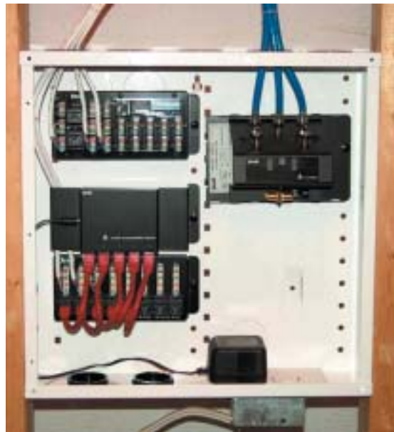
Networked Apartment Communications Gateway™
